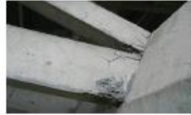
(n) damage mode of the ribs
