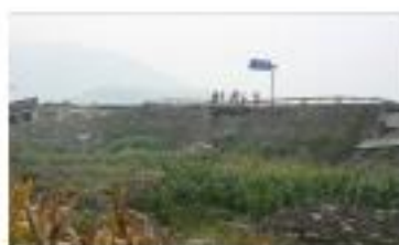
(b) fault rupture went through culverts
