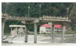
(h) flexure crack
