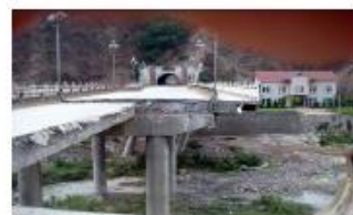
(f) damage of the frame
