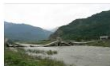
(c) collapse of 2 spans(South)
