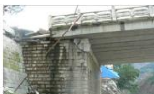
(j) damage of the abutment
