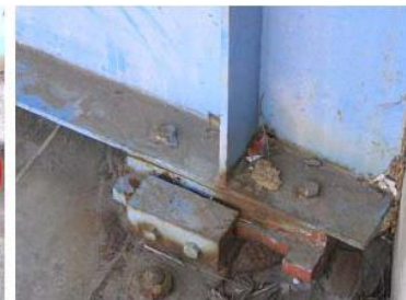
Abnormal gap (movable bearing)
