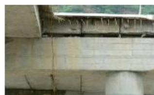
(i) shear crack
