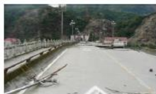
(e) damage of the road
