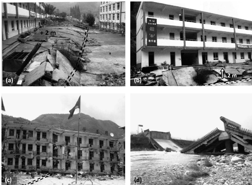
Fig. 1. Examples of reverse fault rupture interaction with structures during the 2008 Wenchuan earthquake in China: (a) the school building on the left was driven 2 m upward, standing on the “moving wall,” and survived the fault-induced deformation practically unscathed; (b) front view of the school building; (c) failure of a three-story building, which was crossed by a fault rupture of 1 m throw; (d) collapse of a bridge span from fault-induced differential displacement of its piers (reprinted with permission from Lin and Ren 2009)
