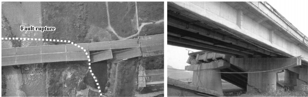
(b) Collapse of two spans and pier shear failure of the Wu-Shi Bridge
