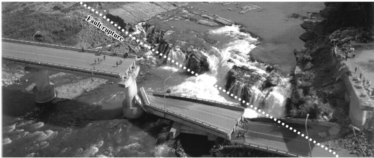
(a) Collapse of two spans of the Bei-Fung Bridge
